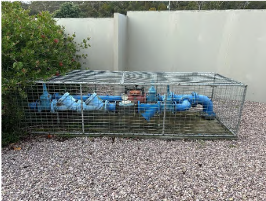
Figure 2: Existing water meter assembly
