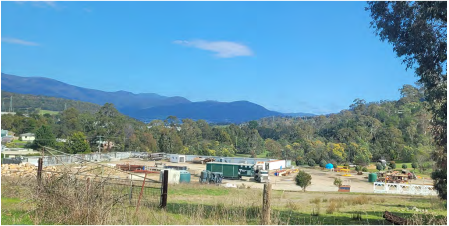
Photo 3 - Storage of materials on 20 Scotts Road, Risdon Vale
